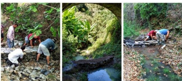
Figure 4. Building 26 deseis in September 2020 in the ravine of Karavas, North Kythera (Images: Rigas Zafeiriou/ MedINA)
